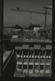
CONSTRUCTION OF GYM EXTENSION Norm McPherson, Marty Hendy and new climbing wall July 1975
